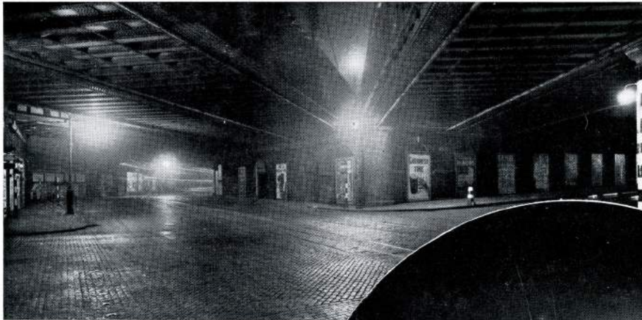
Railway Arches near King's Cross Station. The installation consists of 250w. Sieray "H" type Lamps in Sussex-Sieray Lanterns.
